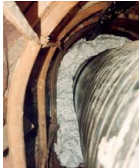
Benefil in the space between the original tunnel and the new lining pipe
