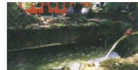
Filling a massive washaway beneath a road on a NSW South Coast roadway
