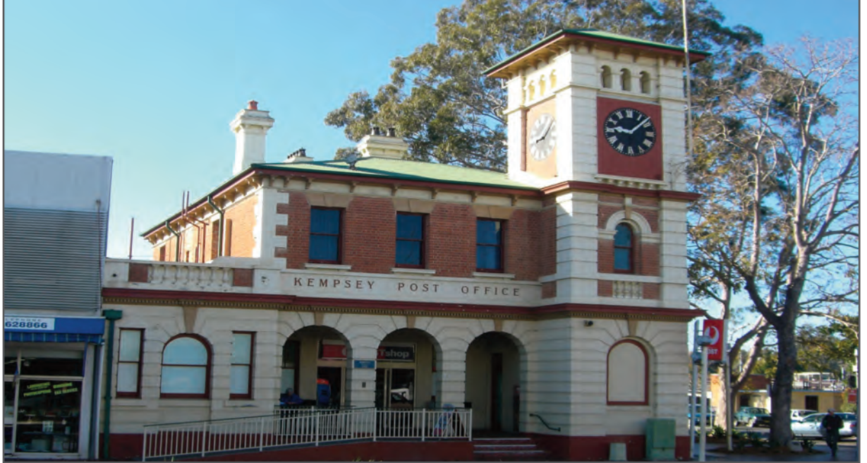
The Post Office at Kempsey, NSW, had been founded on poor fill and subjected to protracted drainage issues, causing long term subsidence with major cracking and distortion of the brickwork across the entire rear section.
