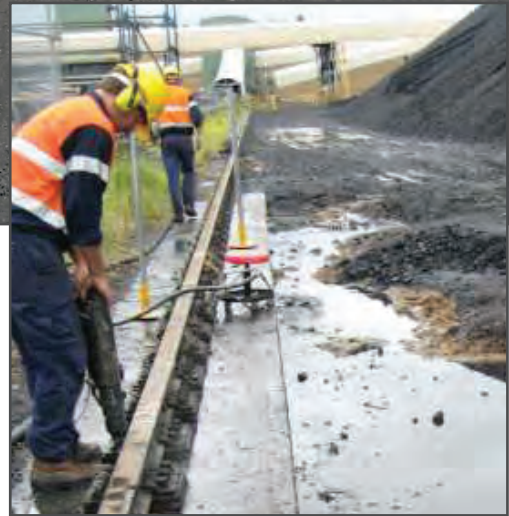
Above: At Rio Tinto's Bengalla Mine in the Hunter Valley, this coal stacker-reclaimer rail had lost support due to excess water ponding beneath the rail slabs. Uretek raised, re-levelled and re-supported the affected areas.
