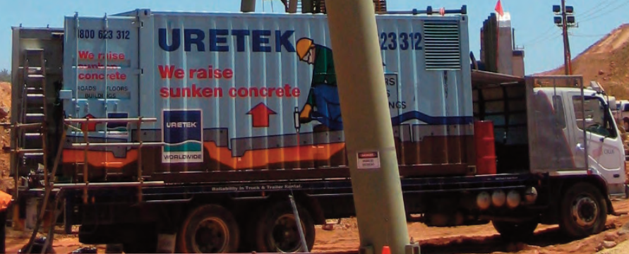
Uretek Ground Engineering re-supporting this two kilometre long conveyor belt system in Western Australia.
