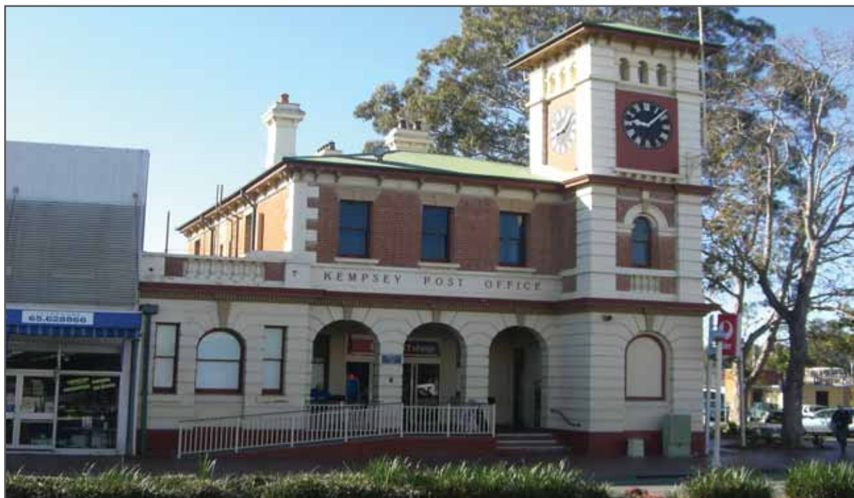
The Post Office at Kempsey, NSW, had been founded on poor fill and subjected to protracted drainage issues, causing long term subsidence with major cracking and distortion of the brickwork across the entire rear section.
