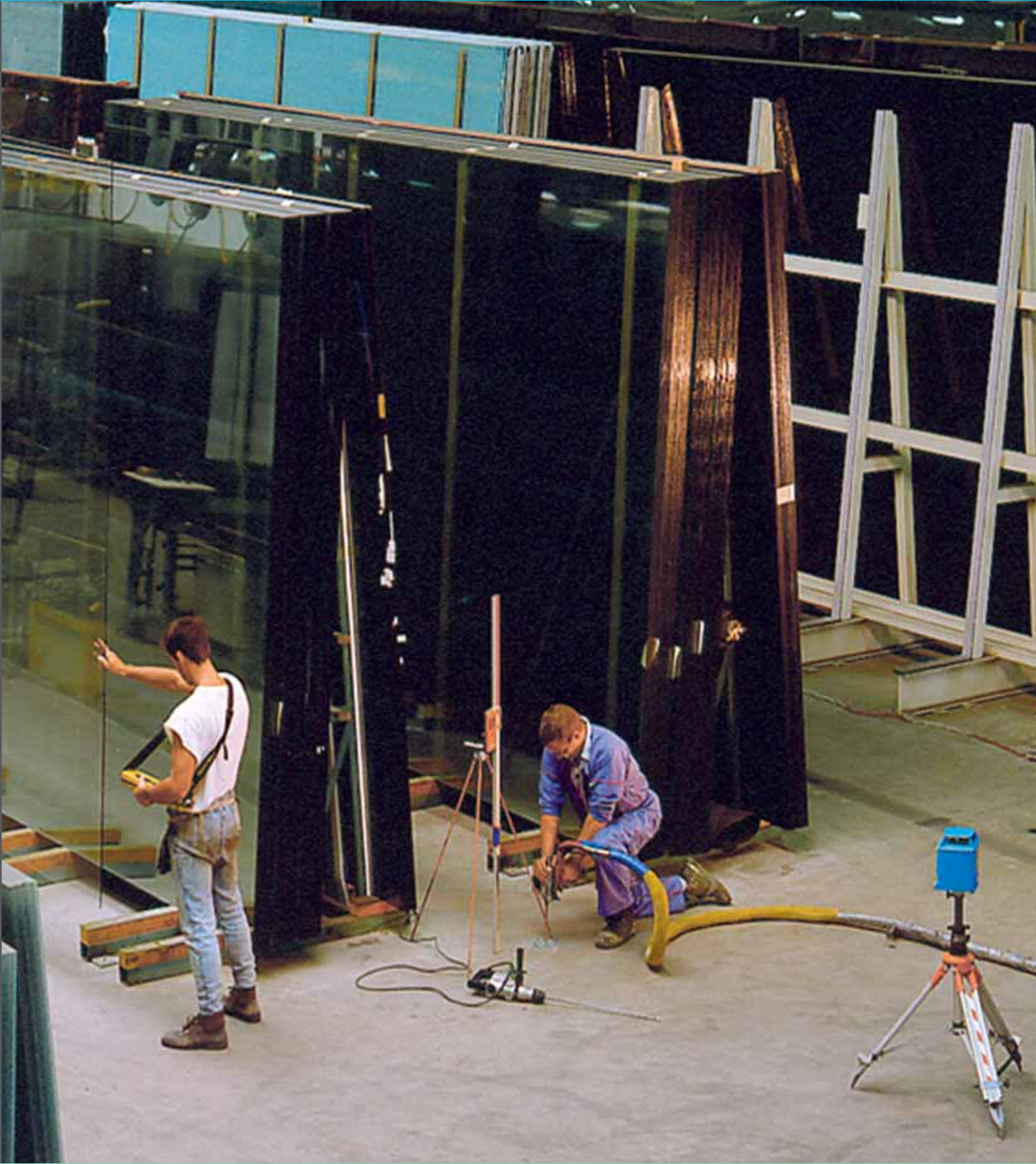
40 tonnes of glass remained in place and normal work continued as URETEK raised and re-supported this floor.
