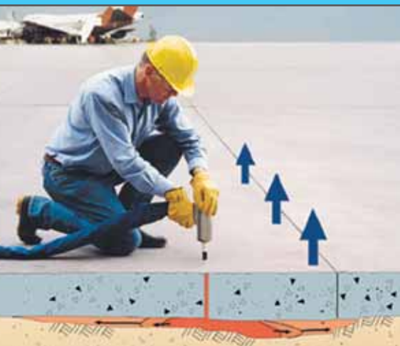
After re-supporting the slab, continued injection raises it, guided by laser level.
