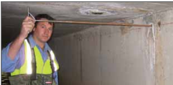
Probing deep voids caused by fines washing away through construction holes and joints in culverts and eroding the sub-base fill under the roadway.
